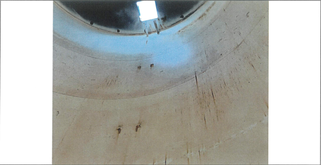
BEFORE Overall view of internal shell with generalized coating failures
