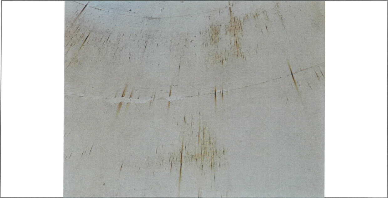
AFTER Zoomed image of coating failures.
